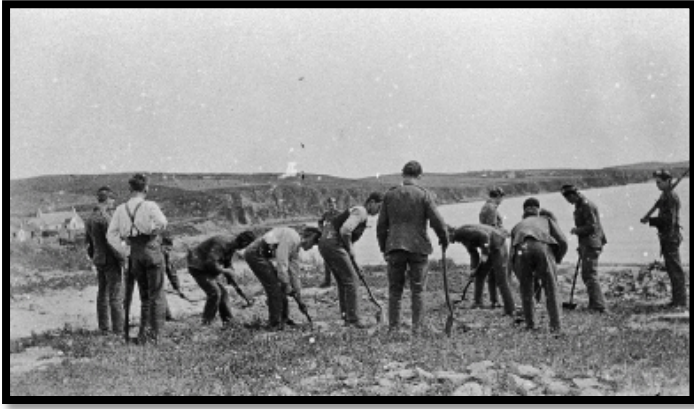
Photo: SM00166 - Sandwich cable guard, digging foundations for something. The cable guards were responsible for guarding the landfalls of the telegraph cable to Shetland, such as Sandwick, Burwick, Belmont.
