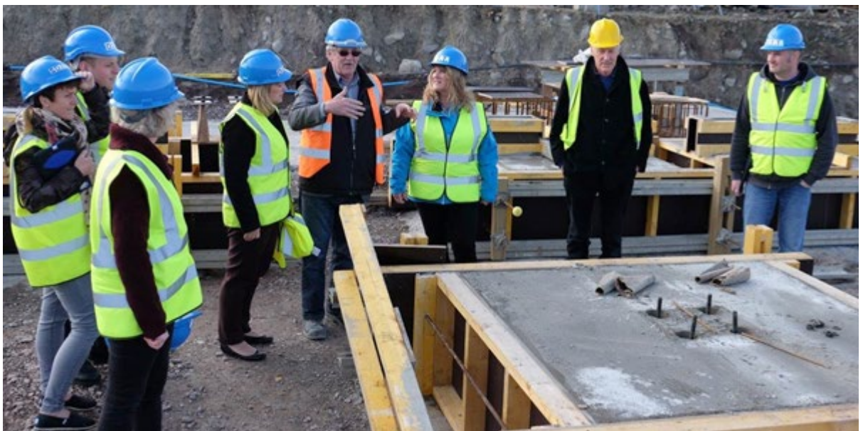
Service users and staff having a project update from the architect and contractor during a site visit at Seafield
