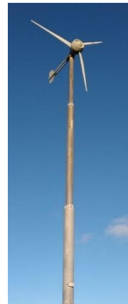
Figure 19 Evance turbine at Bridge End Hall
