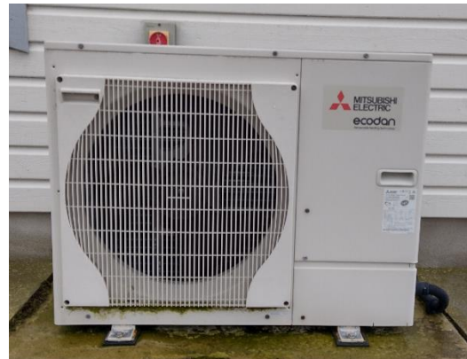
Figure 17 Air source heat pump external unit
