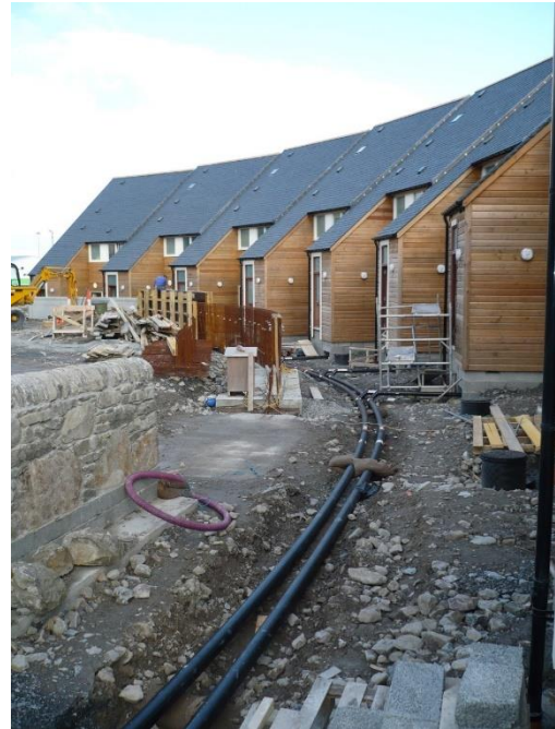
Figure 13 District heating pipes at Da Vadil Lerwick, heat supplied by the Energy Recovery Plant, picture from Shetland Heat Energy and Power.
